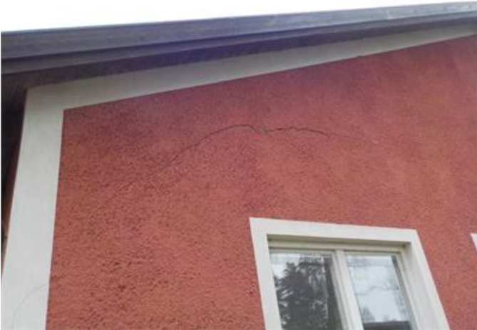
Spricka i fasadputs.
